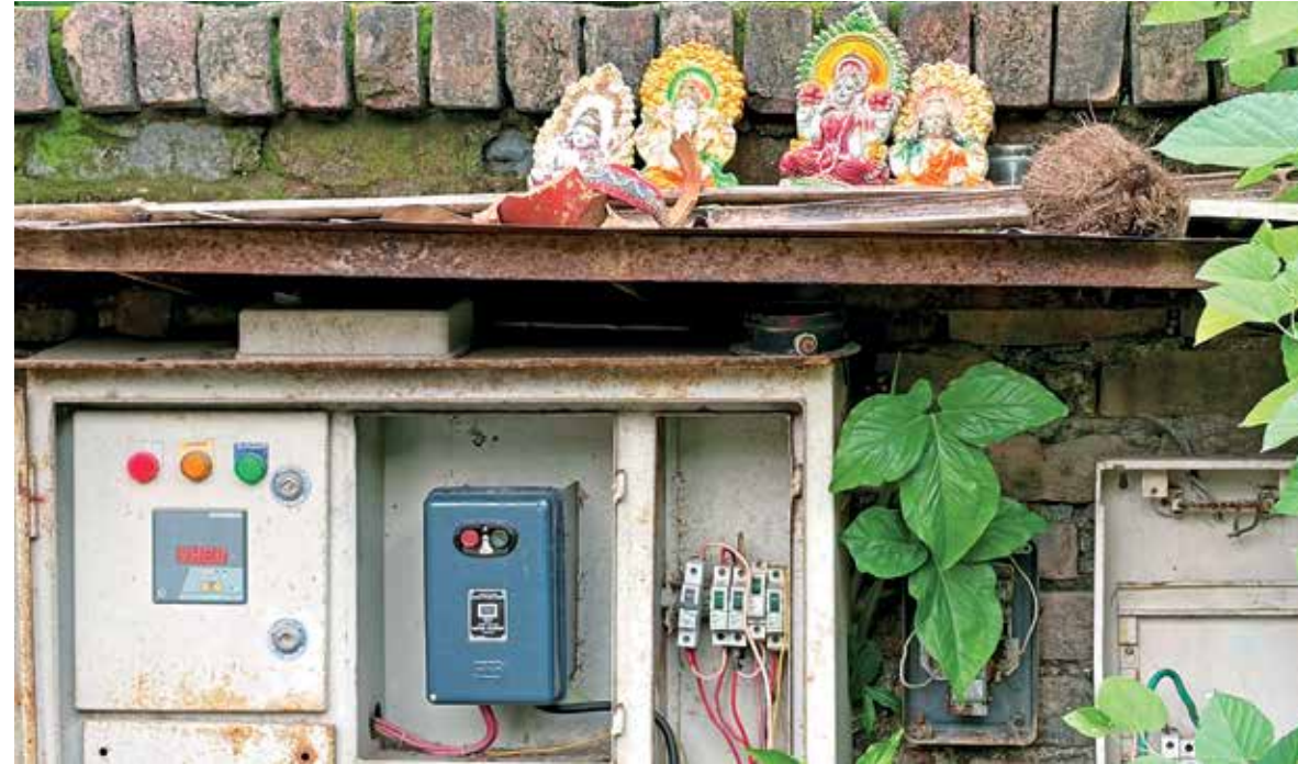
Images of deities adorn exposed electricals in mishap-prone Gurugram
