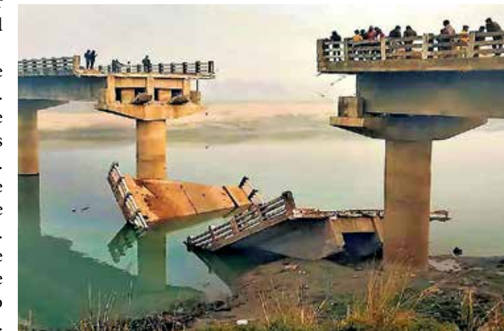
One of the bridges which collapsed in Bihar
