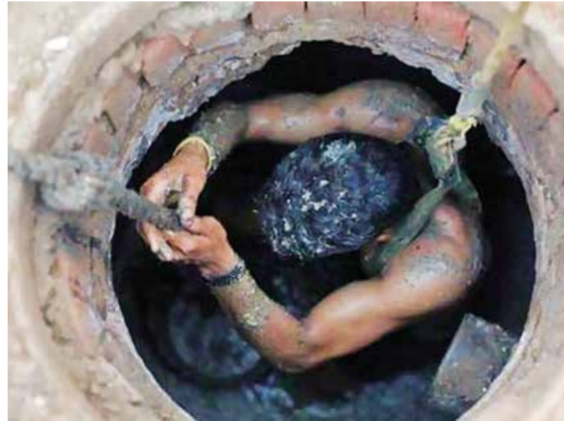
Dalits continue to be sent into manholes
