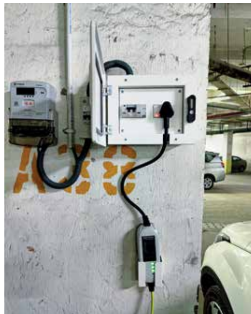
A home charging point is installed for free. Abhinav's is connected to the electricity meter of his flat
