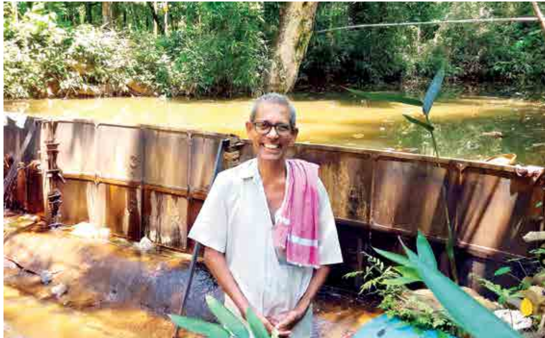
Jogibettu Govinda Bhat, a farmer, with his unique check dam built with mild steel sheets
