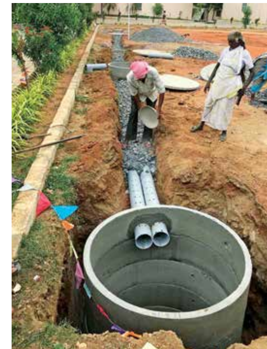
A school in Erode gets a water recharge system
