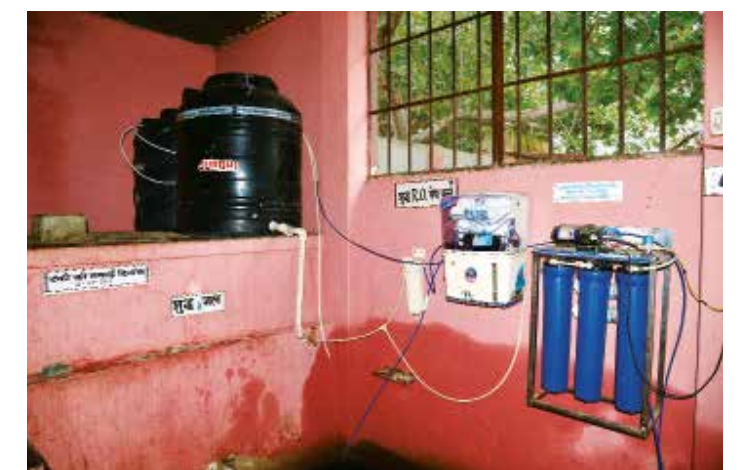
The school has an RO system
