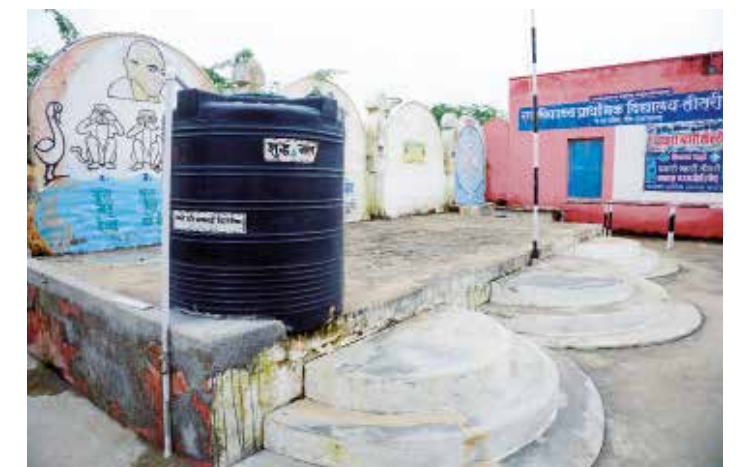
The school's rainwater harvesting system
