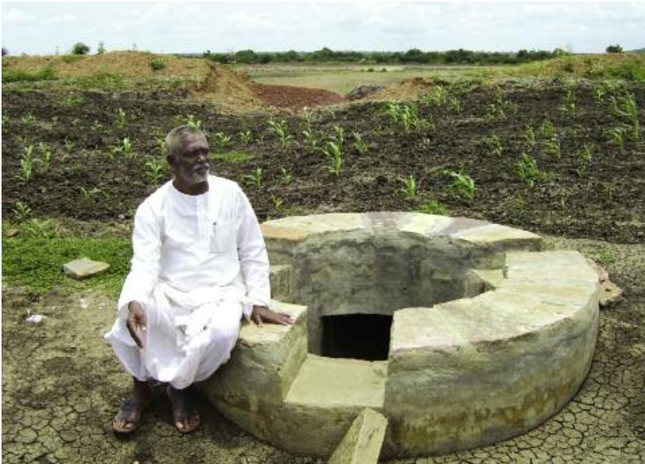
Mallanna Nagaral near a drop inlet spillway. Run-off from the upper fields will bring topsoil and fill the land around this structure.
