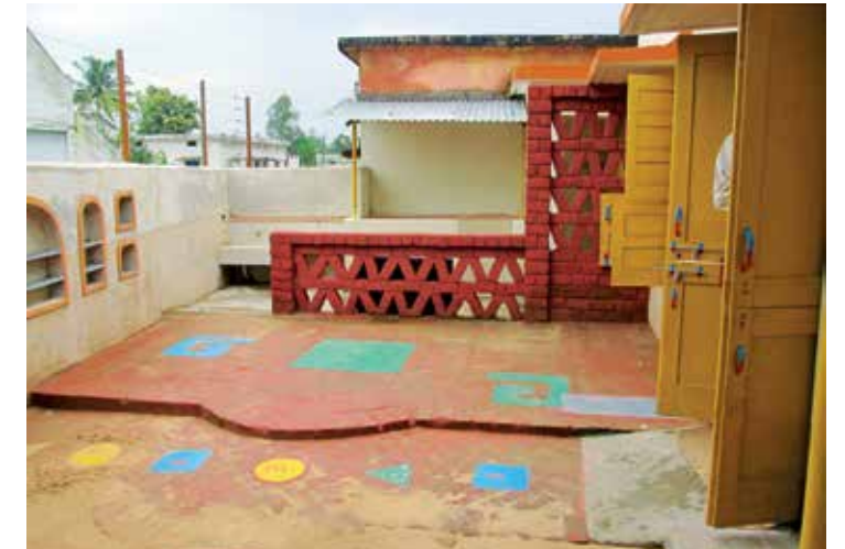
Well-used and child-friendly open spaces are important in an anganwadi. These before and after images show the difference that can be made
