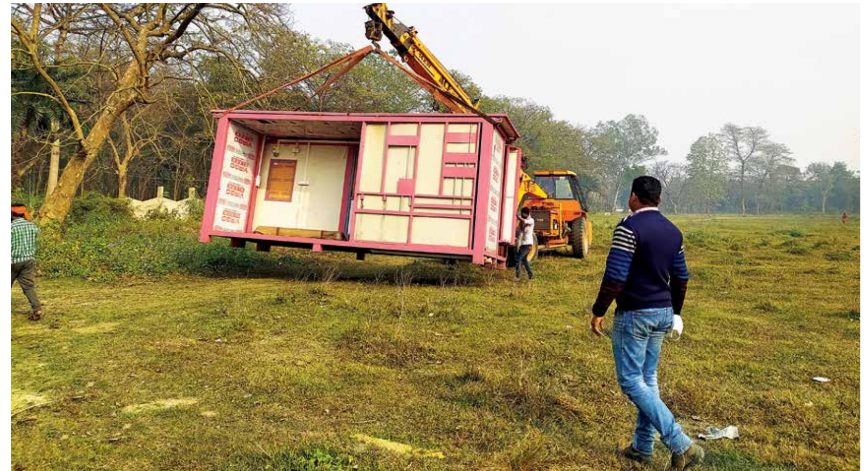
Innovations abound: The first structures for a cancer hospital in Muzaffarpur arrived on a truck from Chennai
