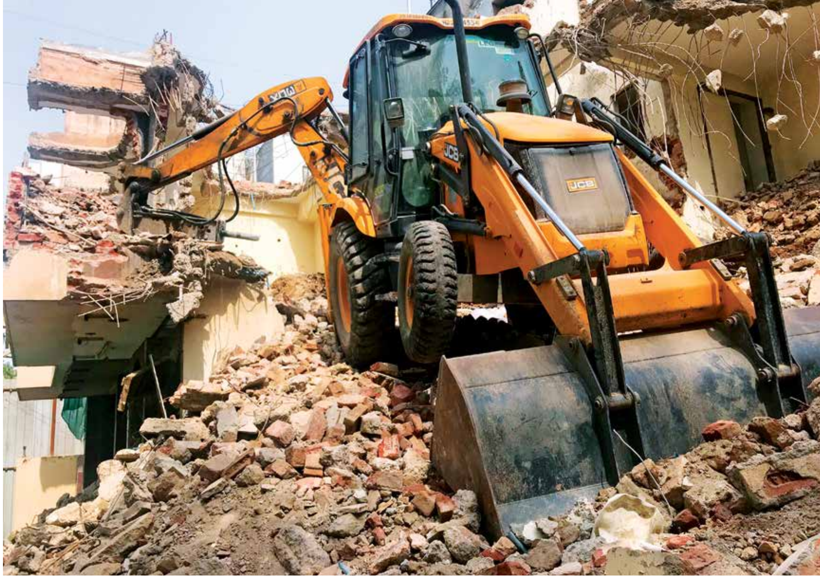
The construction and real estate sector is suffering a steep deficit of 30 percent workers
