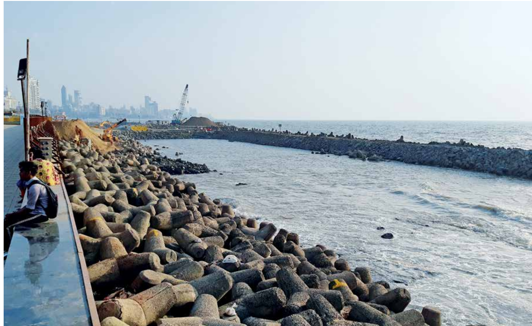
The coastal road will be built entirely on reclaimed land from the sea
