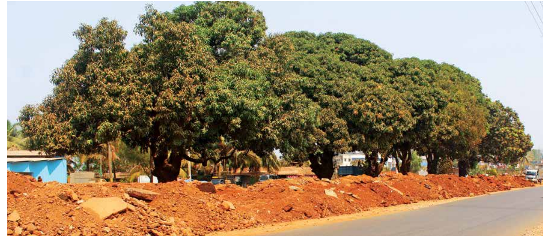
The six mango trees on a road that's been dug up
