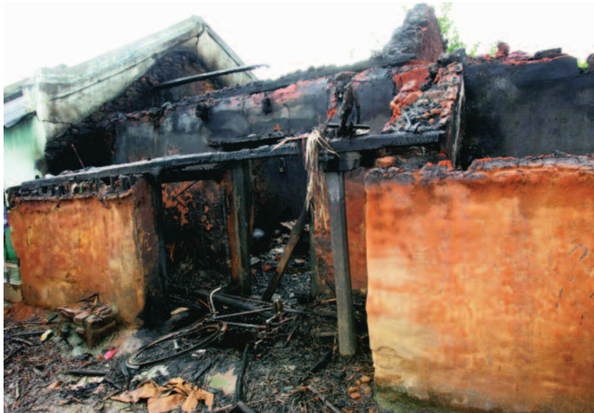
A burnt house
