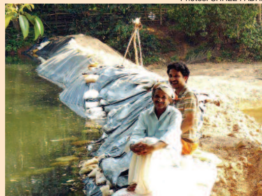
Check dam with sand in plastic sheet
