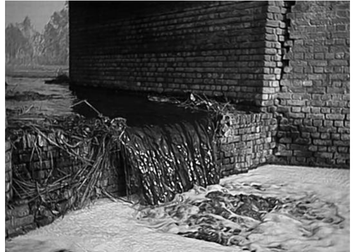
Untreated waste water being released into the Hindon river
