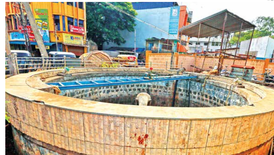
The Khanjar Galli well was repaired in 2010-11 and now supplies water to 12,000 people
