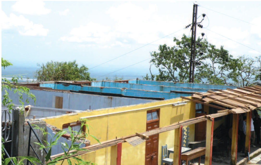
Buildings were devastated
