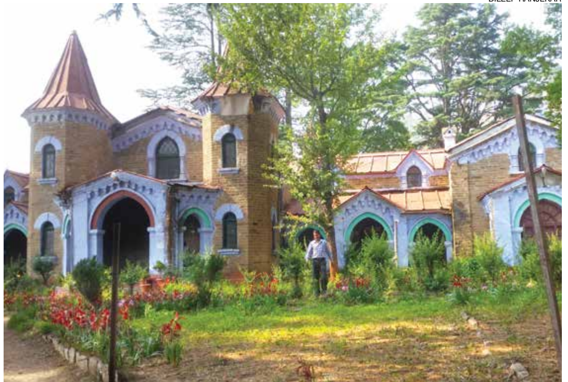
This DIET is housed in a heritage building that is crumbling since it can only be touched by the Archaeological Department
