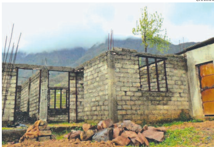
A primary school without a roof in the border district of Poonch
