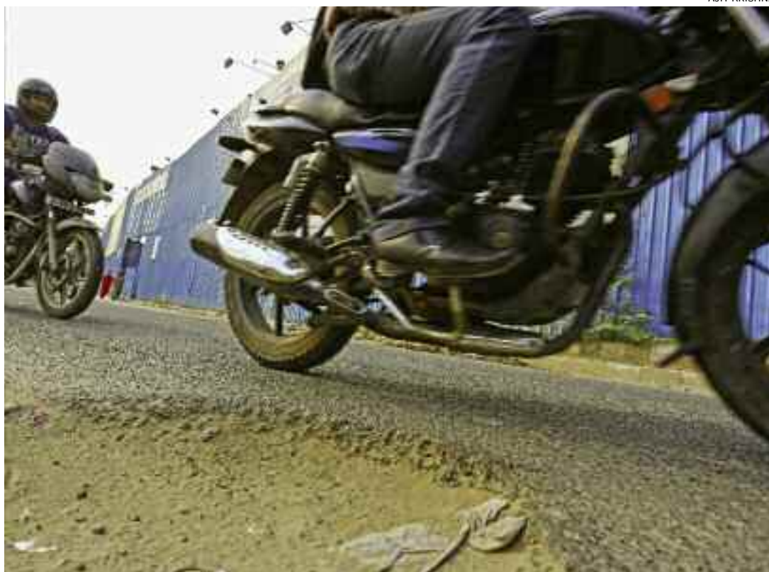
Water collects and creates potholes on poorly constructed roads
